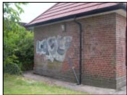
A start has been made to clean graffiti from the Pavilion
